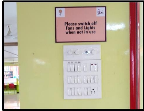
Signages near switch boards
