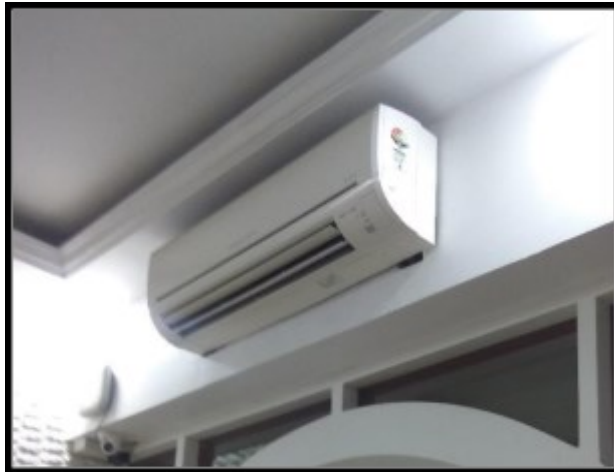
Air Conditioners Installed in Lab
