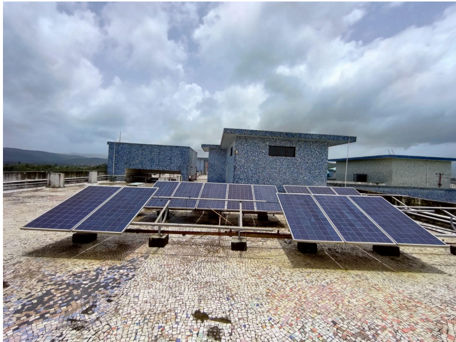
(Solar Panels installed on Rooftop)
