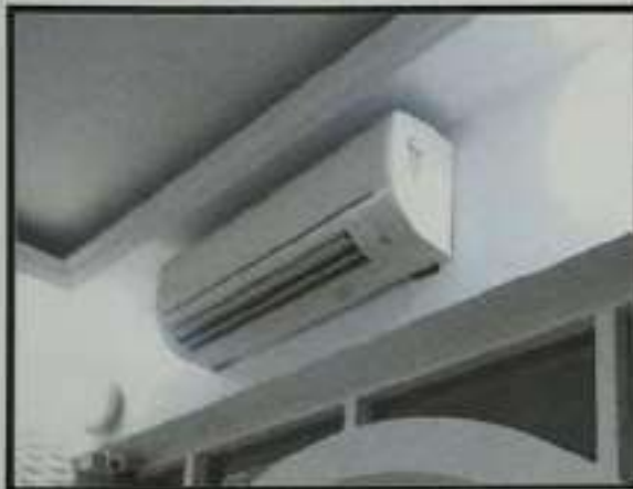
Air Conditioners Installed in Lab
