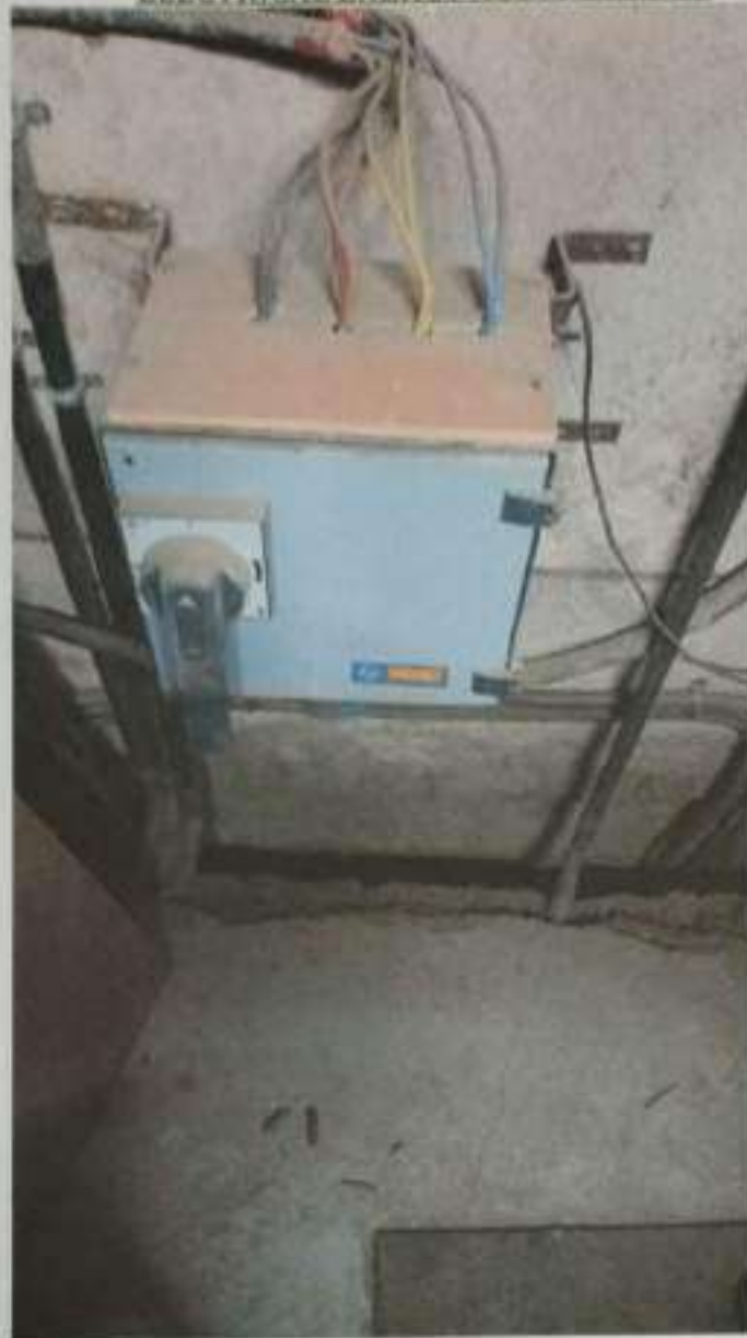
Electrical Insulating mat is provided on flooring.
