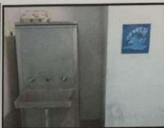
Signages near Cooler/Purifier
